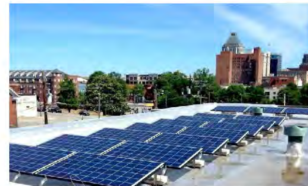
Rooftop solar panels can help achieve Missoula's renewable energy goals.
