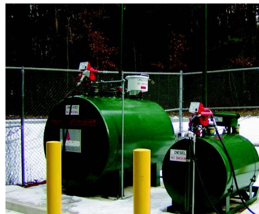
These ASTs are mounted on level impermeable ground with barriers to prevent vehicle collisions. Photo credit: Purdue Extension.
