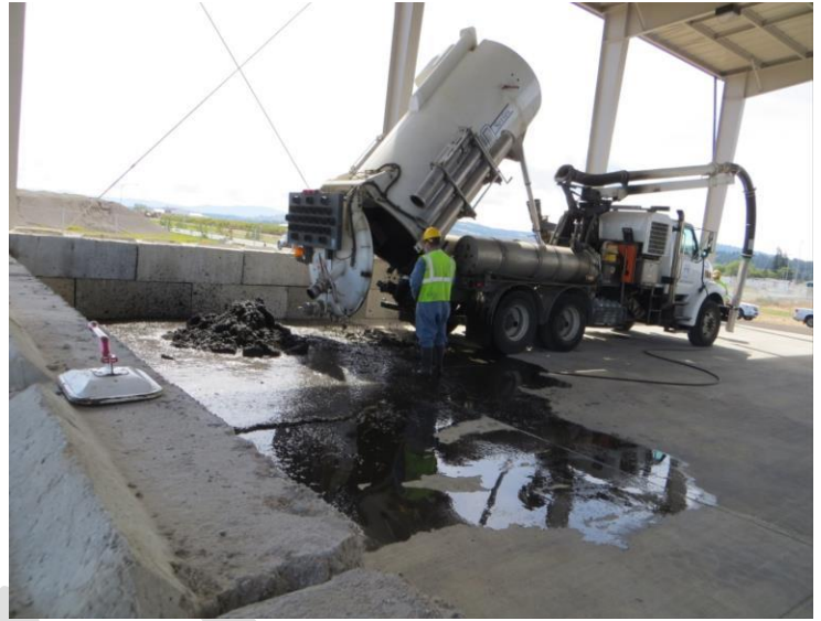
Dewatered materials drain into adjacent settling pool. Water from pool then passes through an oil/water separator, followed by a sand filter bed, and then to a bio-infiltration pond. Photo credit: City of Spokane Decant Facility
