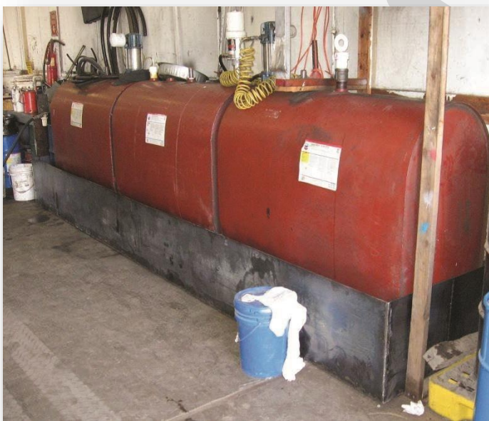
Steel containment for motor oils. Photo credit: Panhandle Health District
