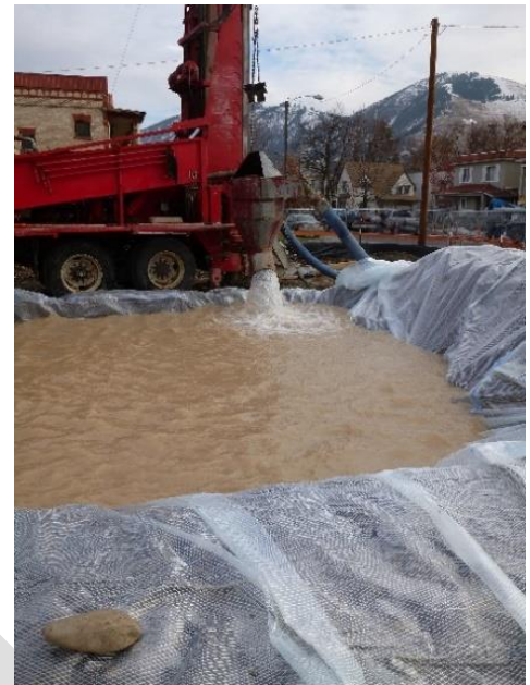
Sediment basin during well development. The rate of filling of this basin exceeded sedimentation. Filtration was necessary prior to discharge to the storm water system.
