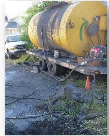
Improper maintenance of asphalt tank and insufficient SOPs for preventing ground contamination
