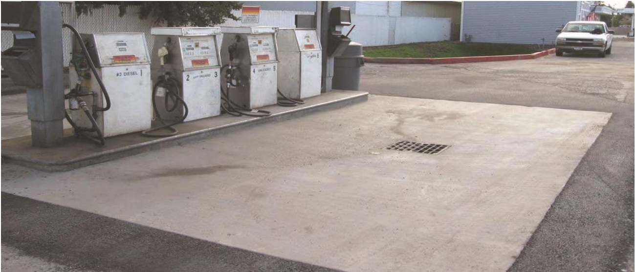
Fueling pad with elevated perimeter to exclude run-on of storm water. Photo credit: Panhandle Health District
