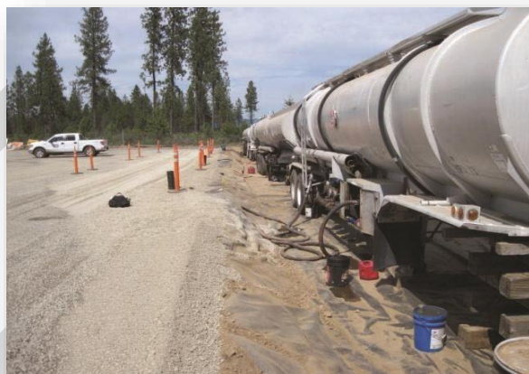
Temporary fueling site with liners under both storage and offload/onload lane (Note black inspection ports along lane). Photo credit: Panhandle Health District.
