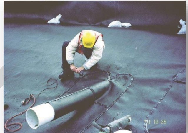
Technician seaming a 'boot' in a liner perforation. Photo credit: Panhandle Health District
