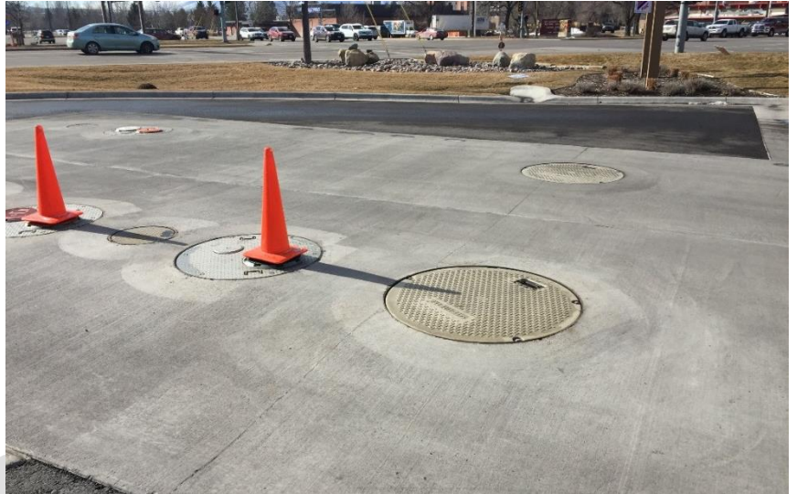
This tank fueling area is graded to drain to a vegetated swale that incorporates a curb cut and beehive grate.
