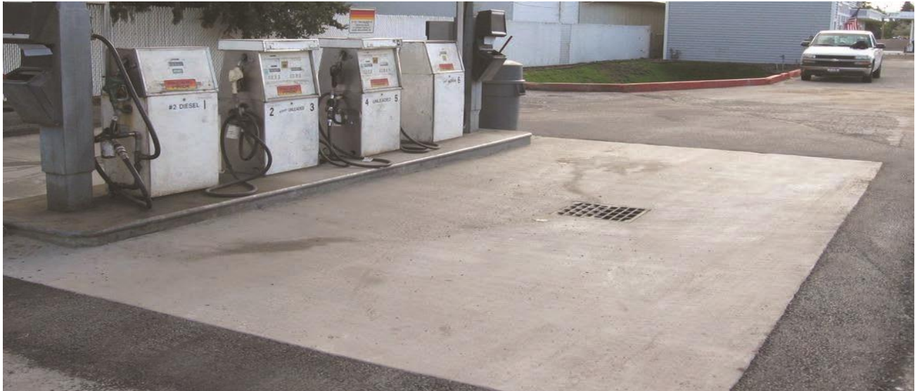
Fueling pad with elevated perimeter to exclude run-on of storm water. Photo credit: Panhandle Health District
