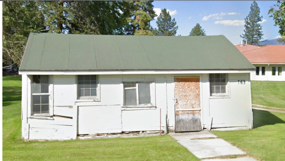
This building was starting to collapse the last time I was at the Fort
