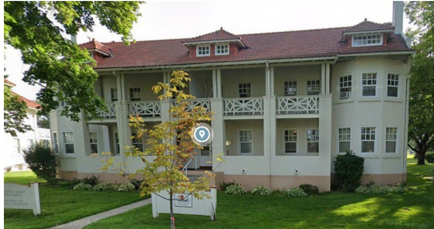
The roof is failing on this building with no owner funds to fix it.
