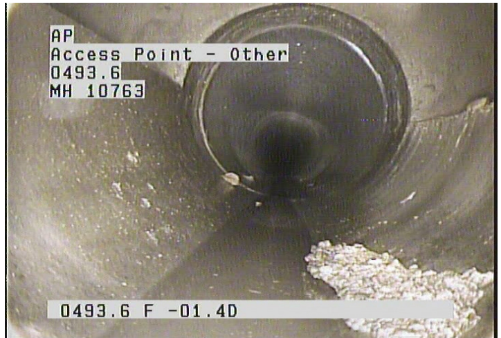
AP - Access Point - Other @ 493.6 ft. MH 10763
