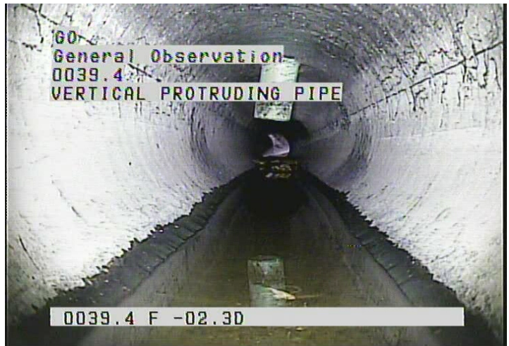
GO - General Observation @ 39.4 ft. VERTICAL PROTRUDING PIPE
