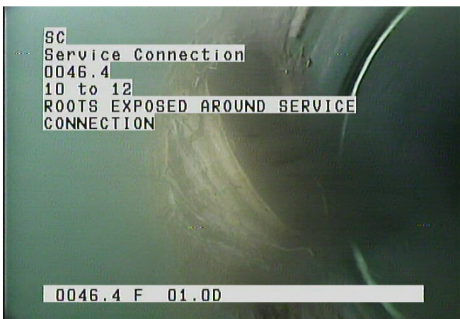
SC - Service Connection @ 46.4 ft. ROOTS EXPOSED AROUND SERVICE CONNECTION
