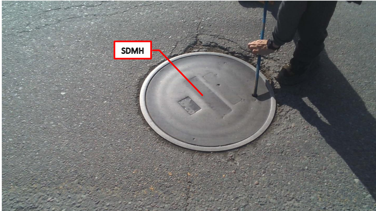
Mainhole Cover (center of lid elevation = rim elevation)
