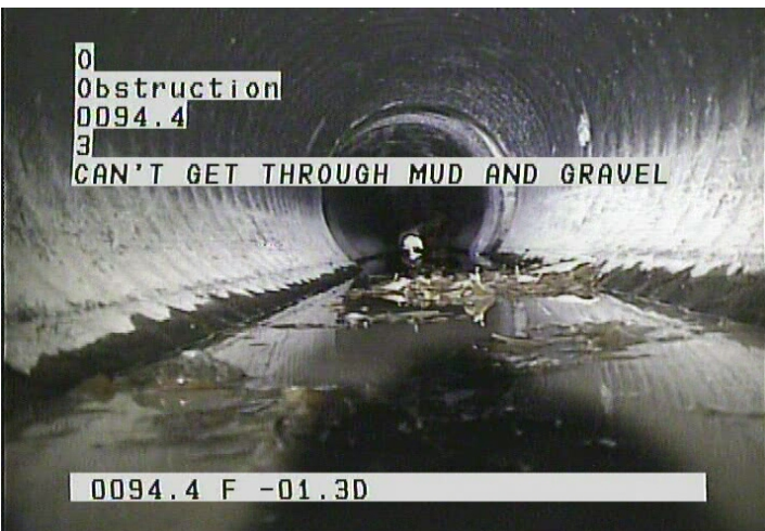
O - Obstruction @ 94.4 ft. CAN'T GET THROUGH MUD AND GRAVEL
