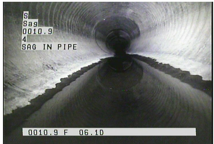
S - Sag @ 10.9 ft. SAG IN PIPE
