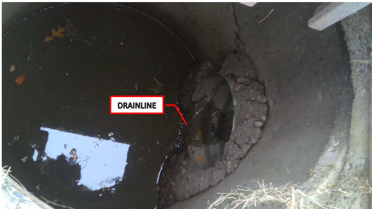
Drainline in Mainhole
