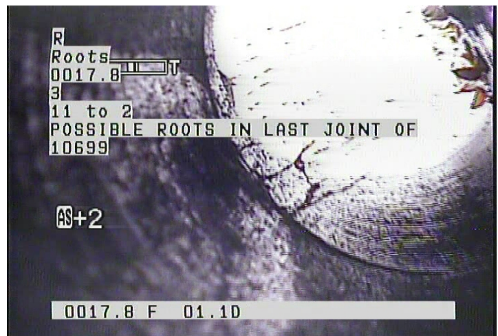
R - Roots @ 17.8 ft. POSSIBLE ROOTS IN LAST JOINT OF 10699
