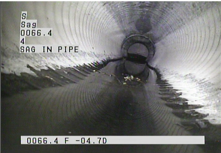
S - Sag @ 66.4 ft. SAG IN PIPE LEAF DAM BLOCKING WATER FLOW
