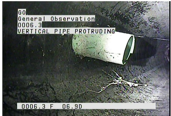
GO - General Observation @ 6.3 ft. VERTICAL PIPE PROTRUDING
