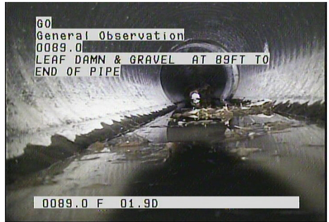
GO - General Observation @ 89.0 ft. LEAF DAMN & GRAVEL AT 89FT TO END OF PIPE
